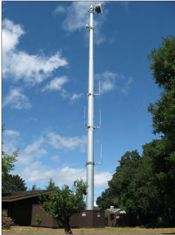
Photo 7 - View of the communications tower that is located adjacent to the south side of the existing Police Station. This tower would be relocated adjacent to the new Police Station under the proposed Master Plan.
