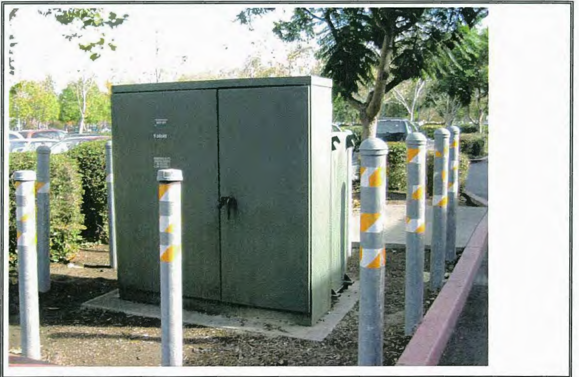
Photograph Number 6 Transformer
